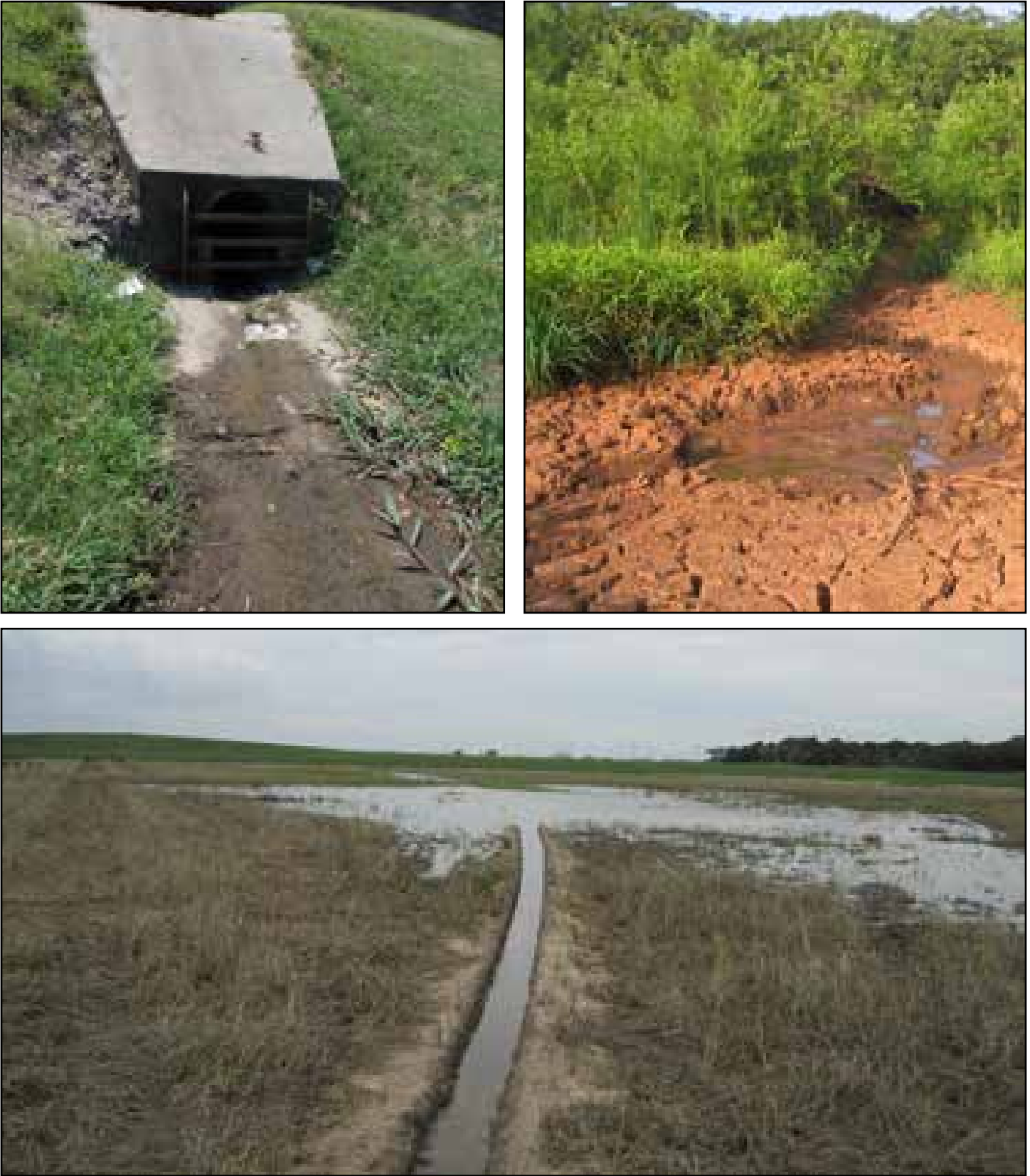
Fig 30. Common stressors that increase hydroperiod: active culvert causing unnatural patterns of filling—major (top left), old pipe culvert that fills wetland during large storm events—moderate (top right), wetland filled by center pivot irrigation (CP) with CP tire track—major (bottom)
